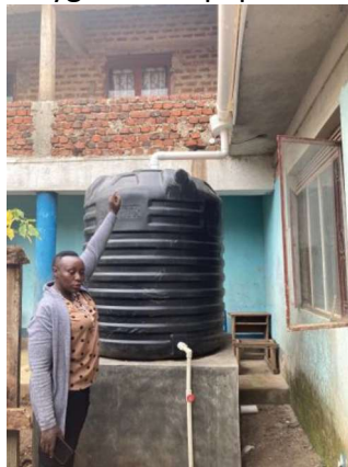
New Water Tank
